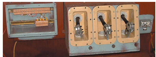
Fig 7 : Typical Termination Arrangement Showing RTD-BTD (L) PSTB (C), Space Heater (R)
